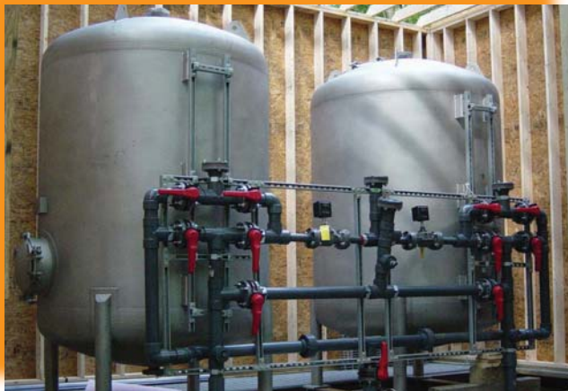
WHITE ROCK WATER CO. (BOW, NH) DEMO SITE - ADI IRON ADSORPTION MEDIA SYSTEM
